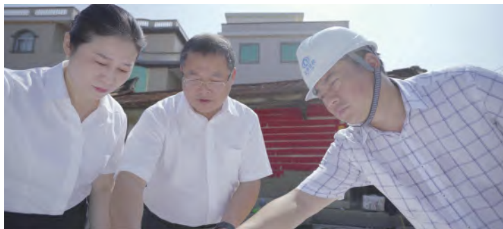
Staff members from Zhangzhou Branch supported the integrated construction of Longhai Water Supply and visited the project site to inspect the progress.
