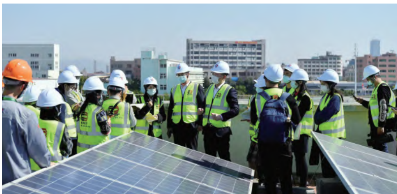
Note: IB supports the construction of Xiamen Lüquan Industrial Roof Distributed Photovoltaic Project.
